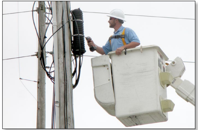
Jared Mobbs, telecom technician, re-installs a fiber optic splice closure. (Photo by Christa Jennings)
