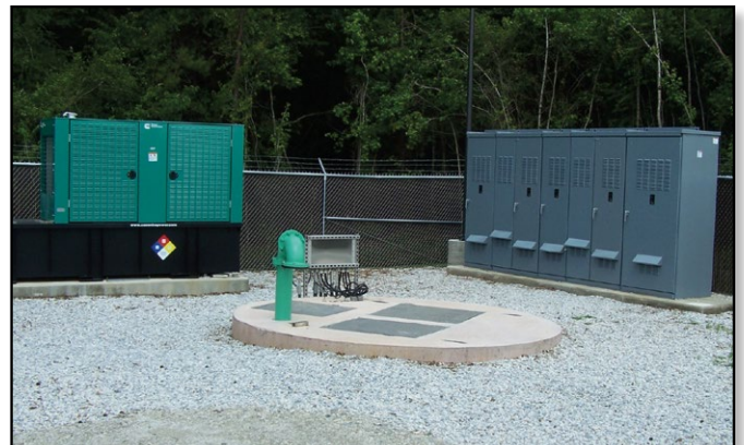
New lift station
