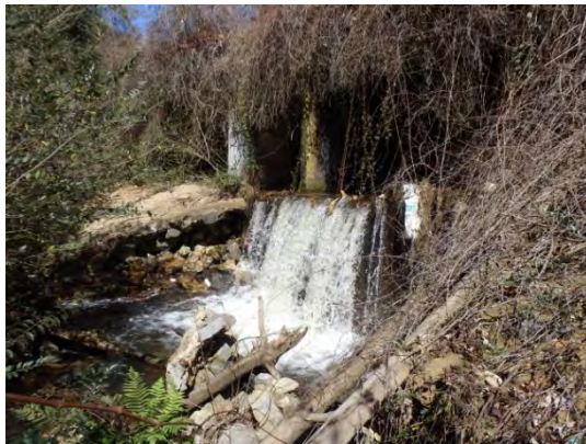
Photo 5. Eroded Culvert Fish Barrier at Highway 98
