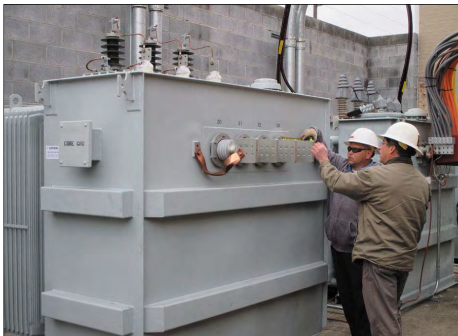
Sylacauga Utilities Board Electric Superintendent Eric Carithers and lineman Jeff Whaley inspect the third transformer.
