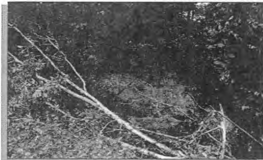
Pictured: Gully wall after collapse from April's catastrophic rain event (Big Mouth Gully, North Section Street). Photo Credit: John Saraceno
