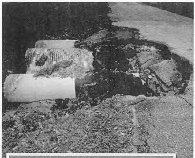
Pictured: Thompson Hall Fire Station Road Washout; Photo Credit: John Saraceno
