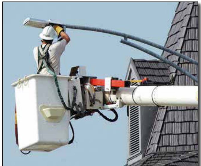
A City of LaFayette Electric Department employee installs one of the city's new LED cobrahead lights on a fixture in downtown.
