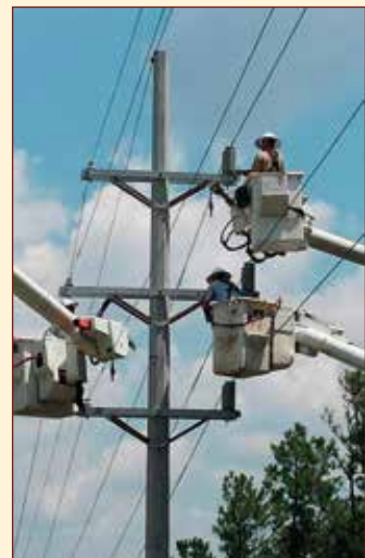
UBT crews replace 14 old wooden poles on 44kV system with new concrete poles and cross-arms.
