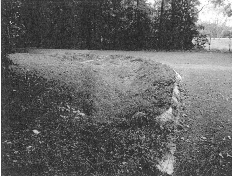
Westley Avenue Bio-retention: Picture taken: December 2013
