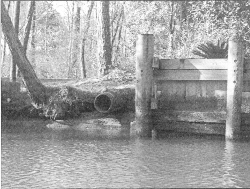
City of Fairhope storm drain pipe into Fly Creek: December 2013
