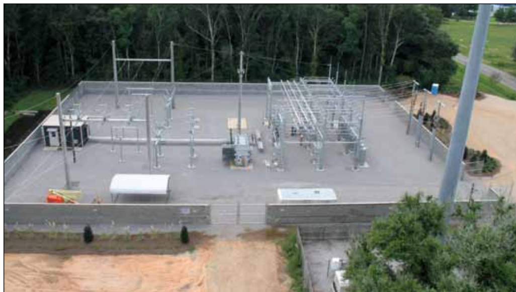
Aerial view of Arthur A. Holk Substation.
