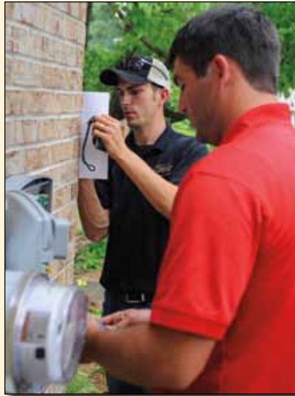
Opelika Power Services crew members, Mikey Hallman and Michael Bass, installing the new system.
