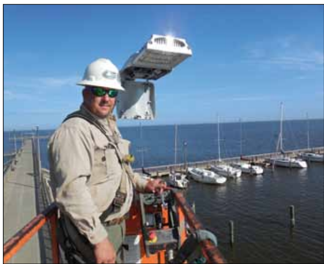
Fairhope Electric Department employee Kevin Wadsworth poses high above the Fairhope City Pier, where he rewired and replaced all the old overhead light fixtures with the new LED lights. (Photo by D. Fran Morley).
