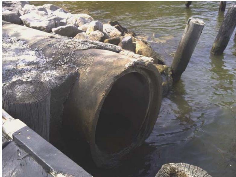
Pictured: South Beach Park storm drain pipe assessed during major outfall assessment—Major Outfall # 12 (December 2012)
