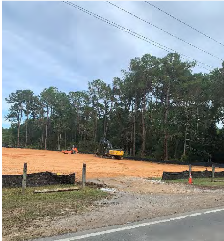
BMP Inspections are conducted by Planning and Zoning Code Enforcement staff initially and as a follow up to ensure BMP minimum requirements are installed and remain installed and effective.
