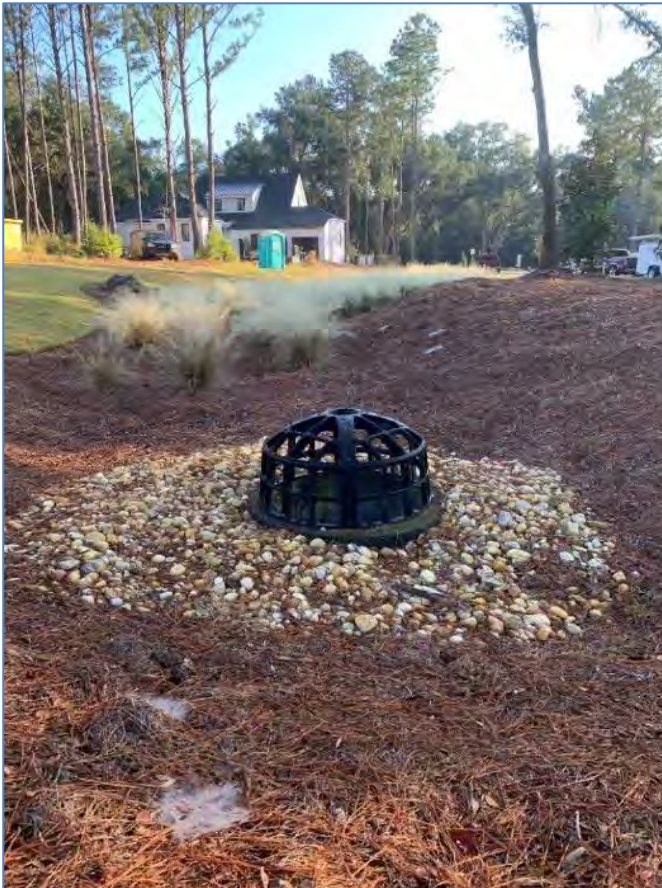
Example of LID used in Hilltop Subdivision, Point Clear Creek watershed. November 2022
