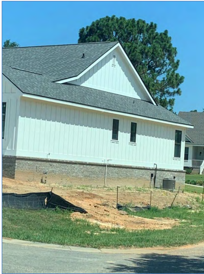
Silt fence maintenance is one of the common comments on a Notice of Violation
