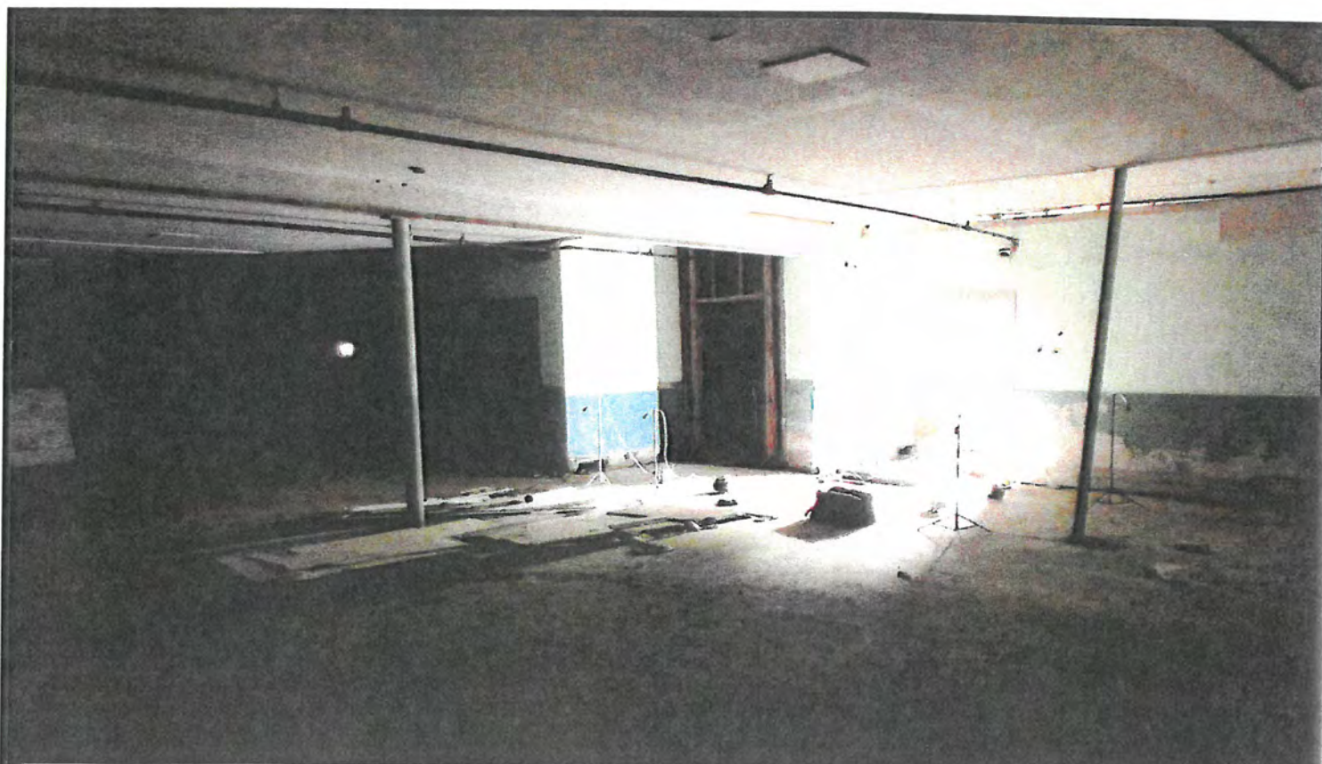
Photo No. 4: VIEW OF THE CENTER WING BASEMENT (UNDER GYM STAGE) AFTER ASBSTOS ABATEMENT.
