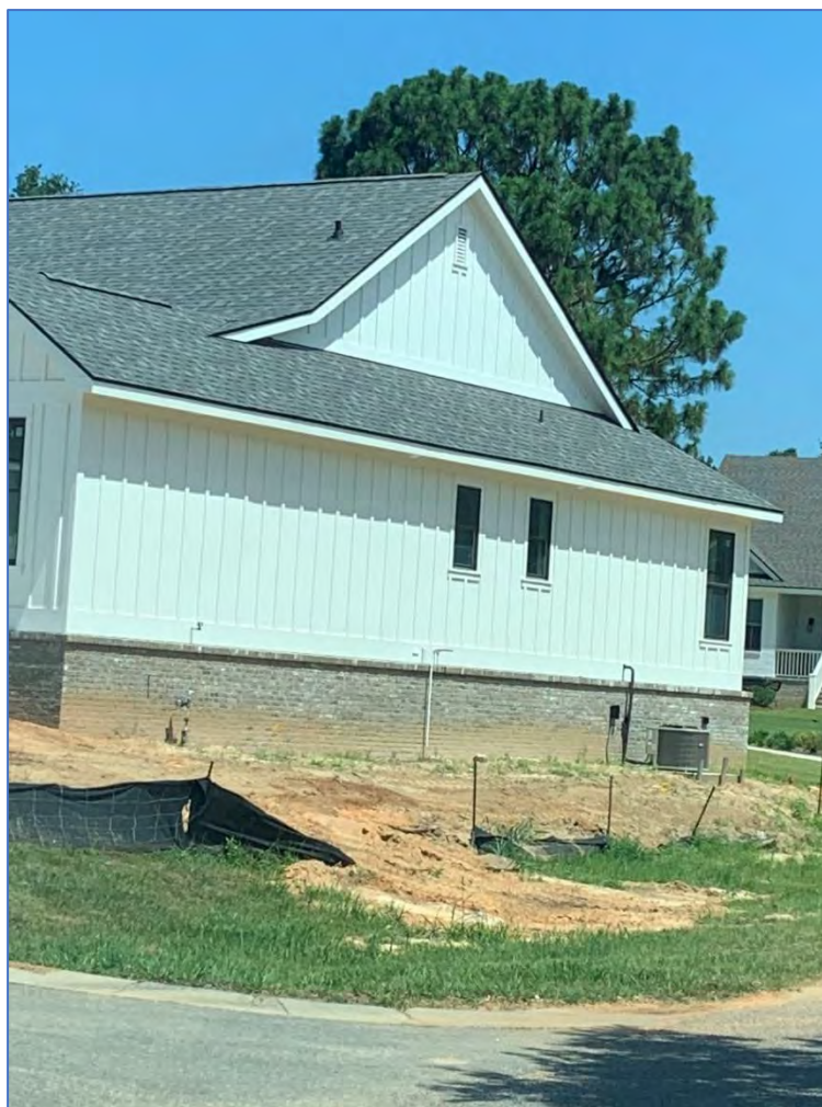
Silt fence maintenance is one of the common comments on a Notice of Violation
