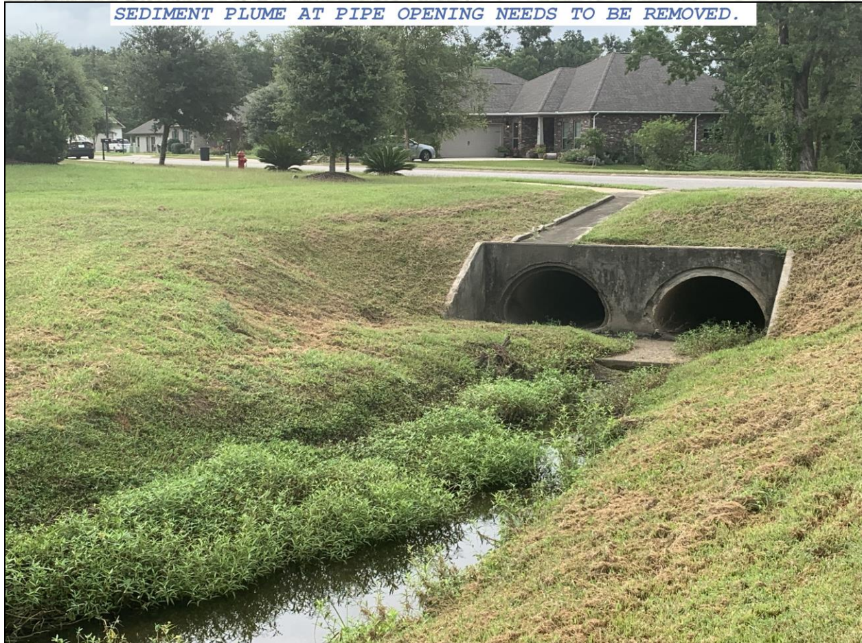
Figure 57 Outfall from 2021 inspection needing sediment removal (Cowpen Creek)
