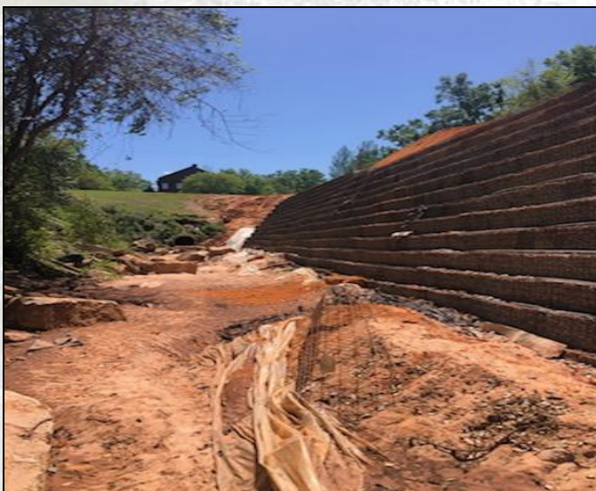
Figure 10 Big Mouth Gully stabilization project (Church and Oak Street) from 2021 continues into the 2022 program period
