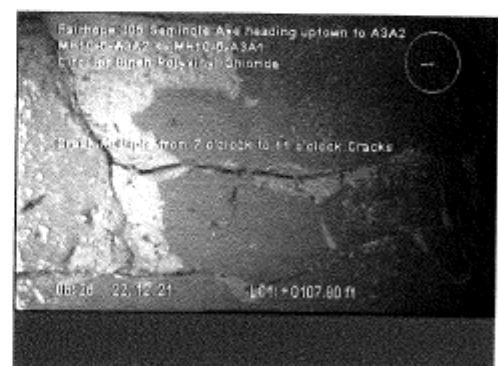
MH10-5-A3A1 to MH10-5-A3A2_d46f84b9-c38b-4a15-9556-f266ee6ba2d3_202 11222_073209_047.jpg, 00:03:03, 107.80ft Crack Multiple from 7 o'clock to 11 o'clock / Cracks
