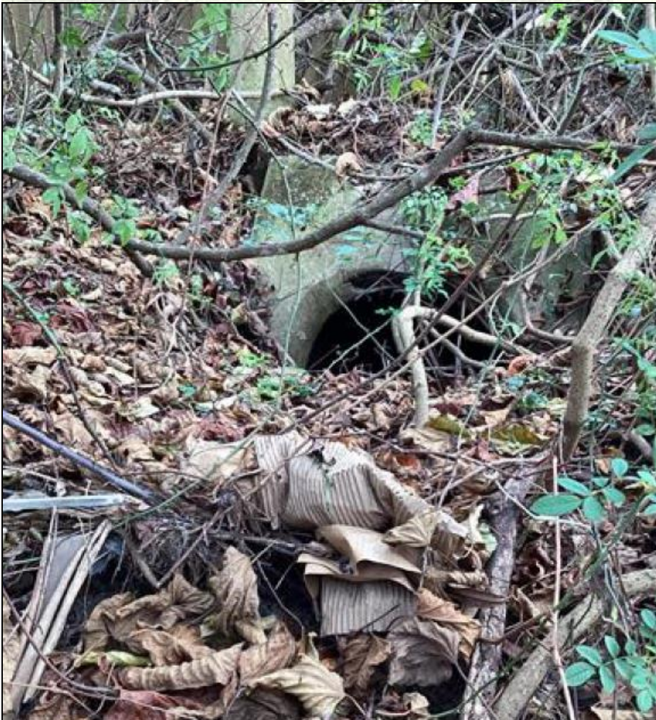
Figure 40 Example of deficient outfall, CC214919a
