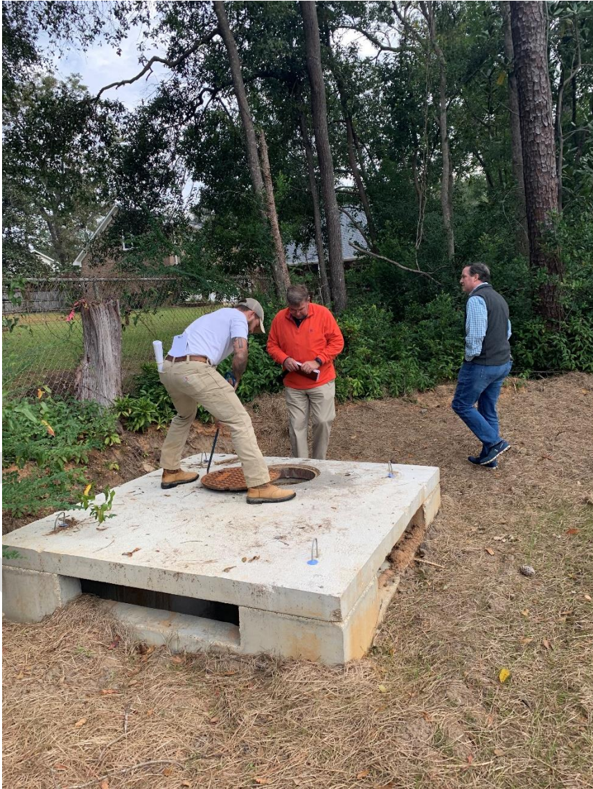
Figure 29: Final Plat Approval walk through inspection Hermitage Court subdivision, Big Mouth Gully Watershed
