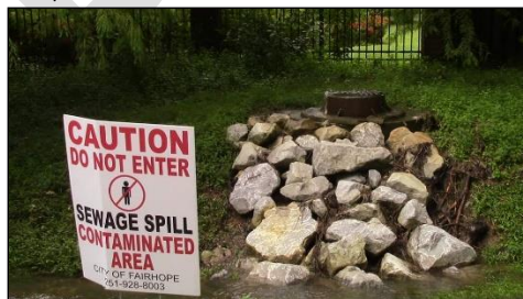
Figure 17 Signage is used to notify the public of areas of sewer overflows (Tatumville Gully)
