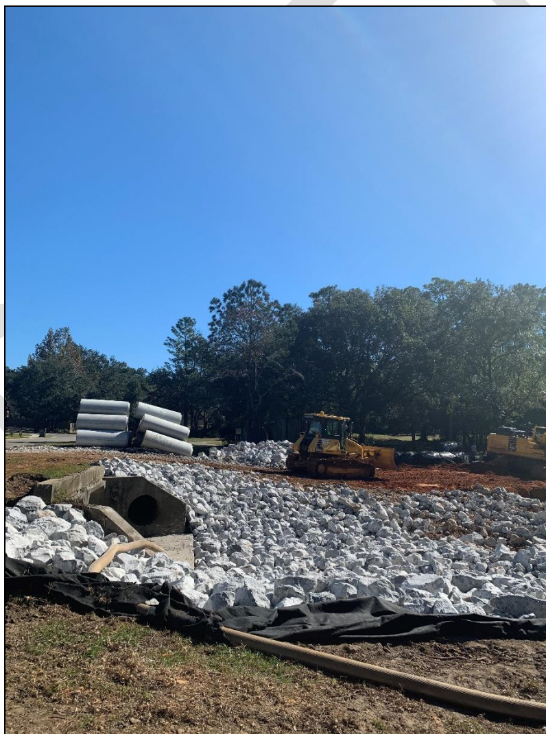
Figure 40: City of Fairhope drainage improvement project at Quail Creek Golf Course, Cowpen Creek Watershed, November 2021
