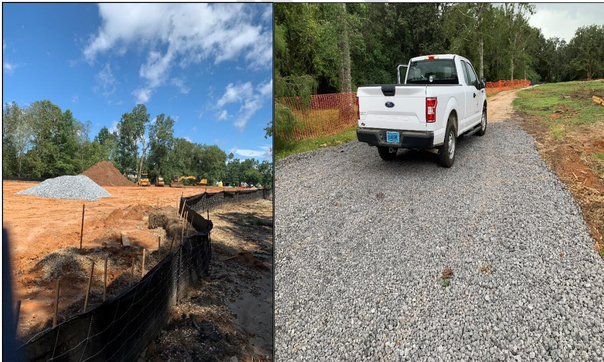
Figure 31 BMP inspection verifying construction entrance and silt fence placement (Substation project, Morphy Avenue, September 2021)
