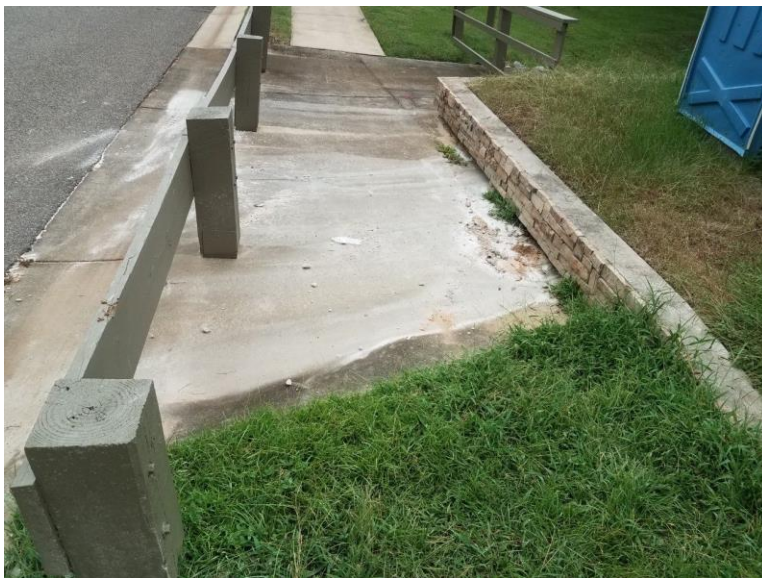
Figure 19 Staining in front of storm drain indicates illicit discharge, Song Grove subdivision, August 2020
