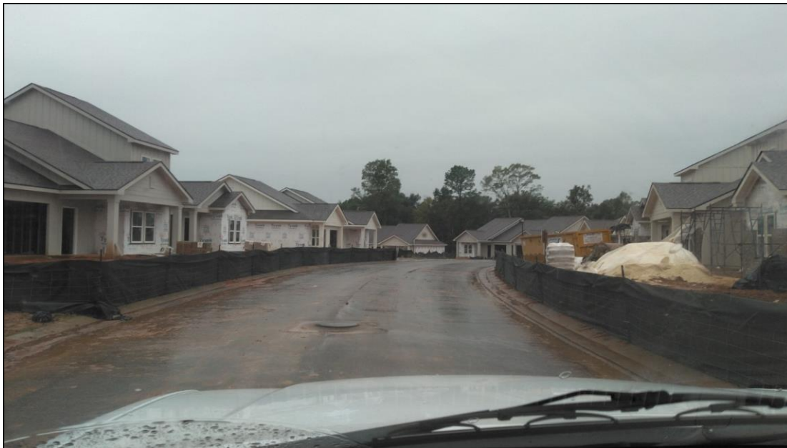
Figure 37 Example of multi-occupancy project underway in 2019. The contractor installed the asphalt binder in advance of vertical construction to meet the new requirement in the City of Fairhope Erosion and Sediment Control Ordinance.
