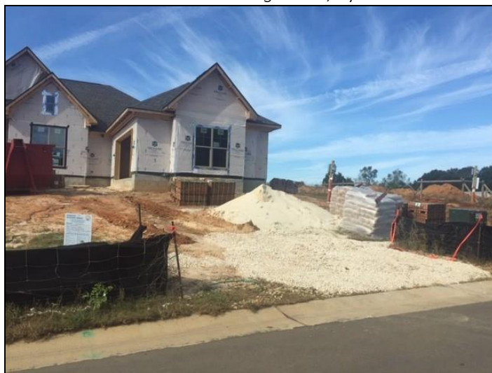
Figure 43 BMP minimum requirements include a silt fence and a construction entrance for residential construction.
