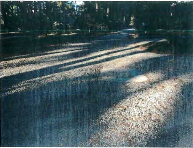
Looking north along N. Mobile Street with new drainage structure in foreground
