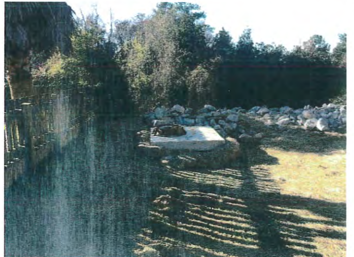
Looking west toward edge of bluff with drainage structure within drainage and utilities easement
