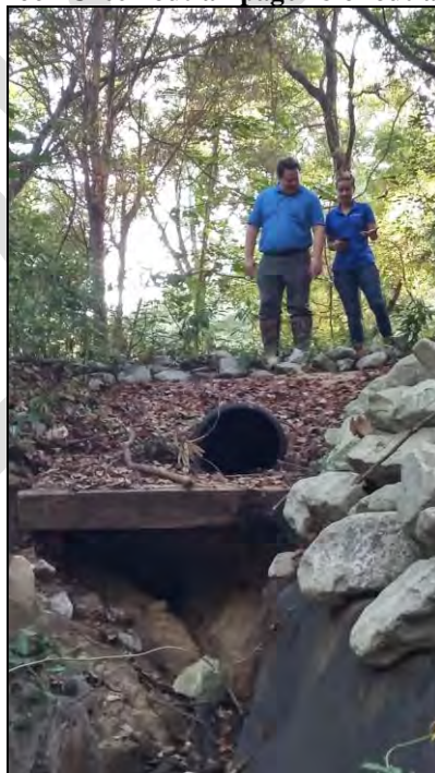
Figure 25 Planning and Zoning staff conduct an assessment of Rock Creek outfall from page 18 of outfall inventory
