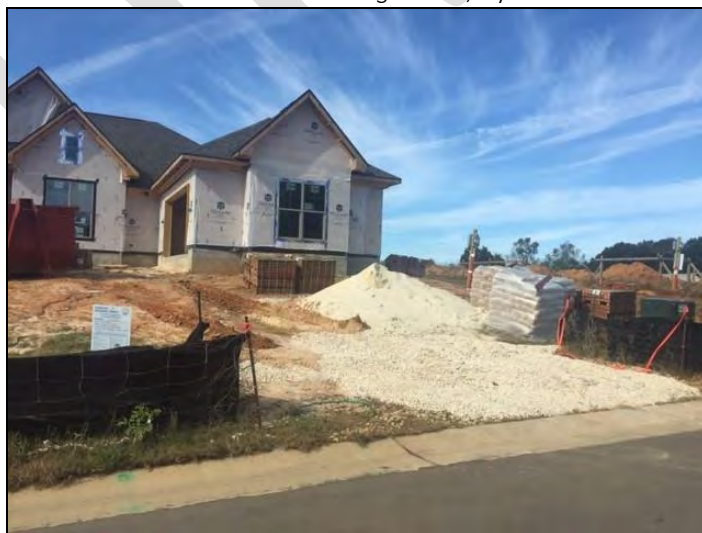
Figure 32 BMP minimum requirements include a silt fence and a construction entrance for residential construction.
