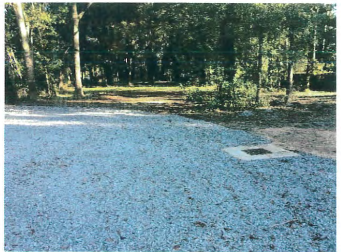
Looking east within cul-de-sac at terminus of N. Mobile Street with new drainage structure at right
