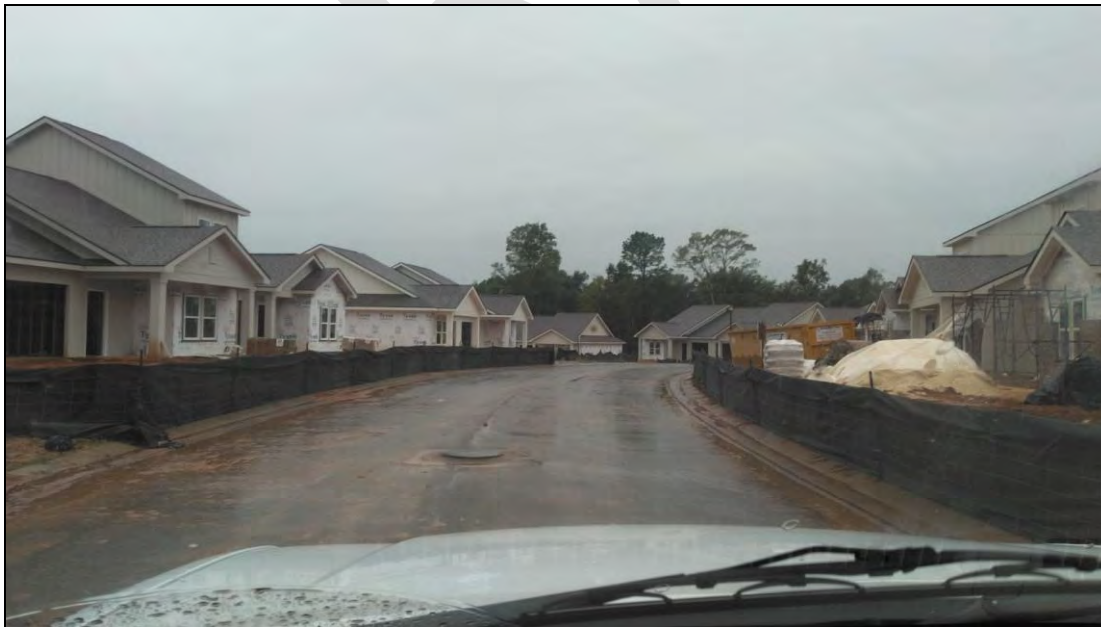
Figure 26 Example of multi-occupancy project underway. The contractor installed the asphalt binder in advance of vertical construction to meet the new requirement in the City of Fairhope Erosion and Sediment Control Ordinance.
