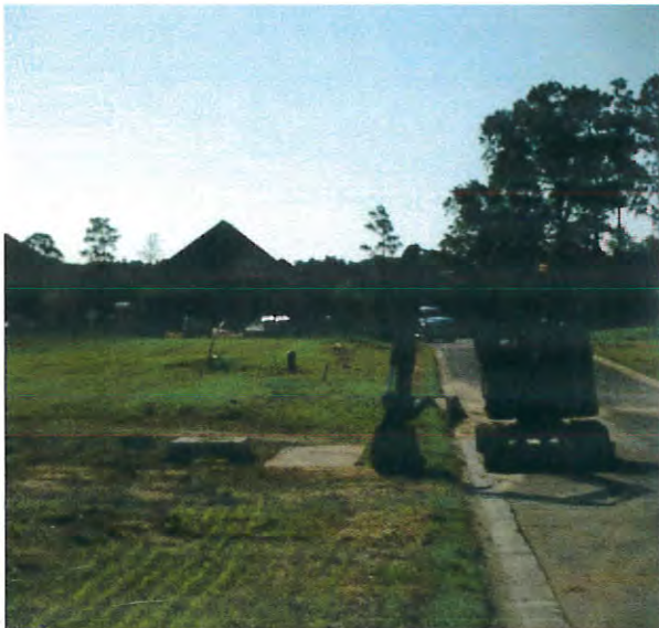
View of inlet requiring repair.
