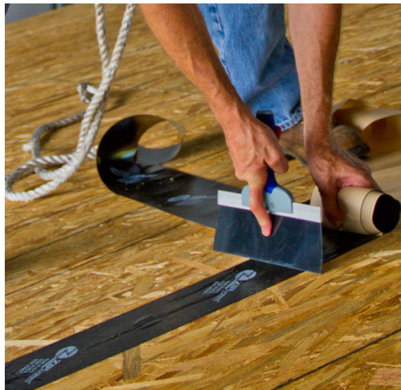
Figure 0-2. Applying qualified tape to roof deck seams using flat blade to eliminate voids and wrinkles.
