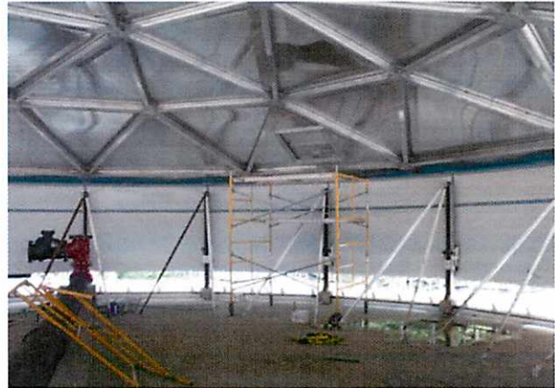
Potable Water with Aluminum Dome
