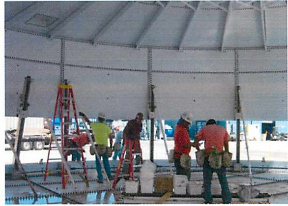
Potable Water with Steel Bottom
