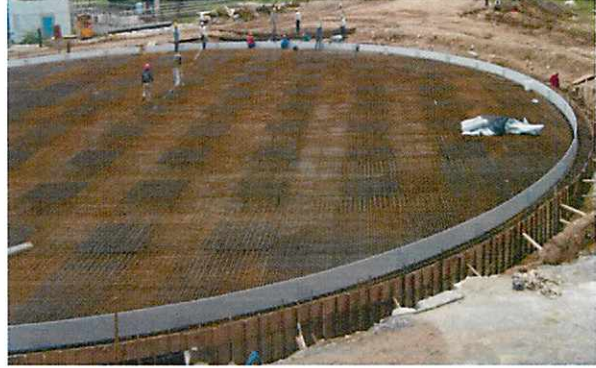
Potable Water Tank - Base Setting Anchor Ring
