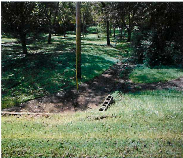
View of drainage going toward Pecan Ridge Sub.
