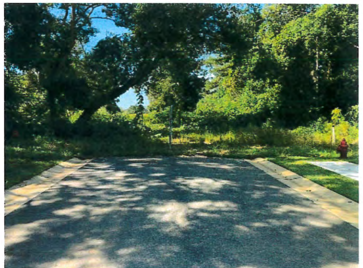
View looking at future connection with Kit Fox Ave SD 18.39 Fox Hollow, Phase III – November 5, 2018
