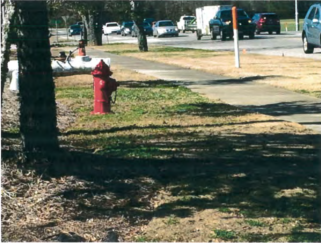
Existing fire hydrant along CR48 near existing medical facility
