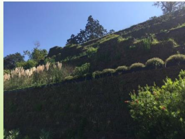
905 Sea Cliff Drive, recent bluff stabilization project appeared to be holding up well
