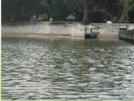
Drain pipe on North side of Orange Street pier did not appear to be discharging at time of inspection
