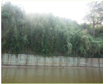
Bamboo is being used for bluff stabilization (Sea Cliff Drive; address unknown)
