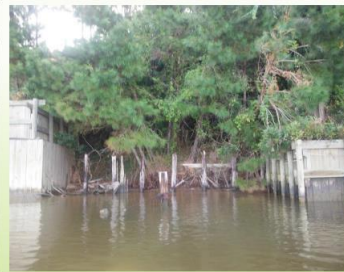
Erosion and undermining of embankment/trees, between two sea walls (Sea Cliff Drive, address unknown but possibly near 917 Sea Cliff Drive)
