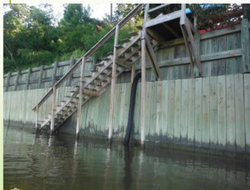
Drain pipe from residential yard: not subject to permitting per Building Official (Sea Cliff Drive, address unknown)
