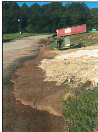
Pictured: Stop Work Order issued to builder with non-compliant site
