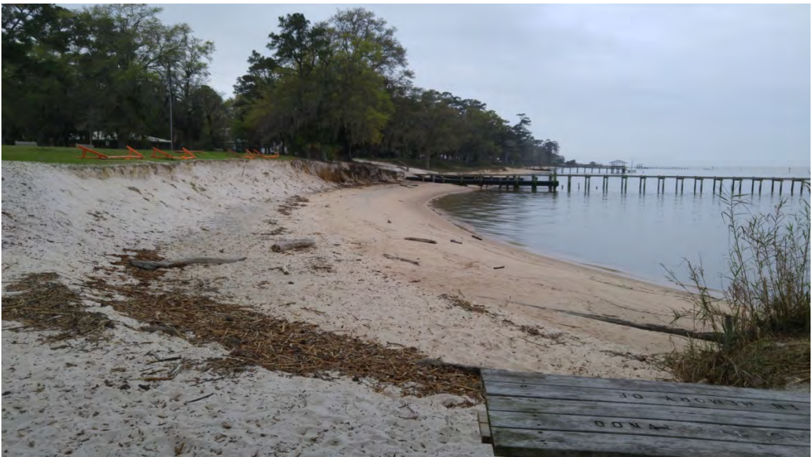
Figure 13: Photograph (facing south) showing winter erosion at the northern end of Magnolia Beach Park, near the boat launch (February 2016).
