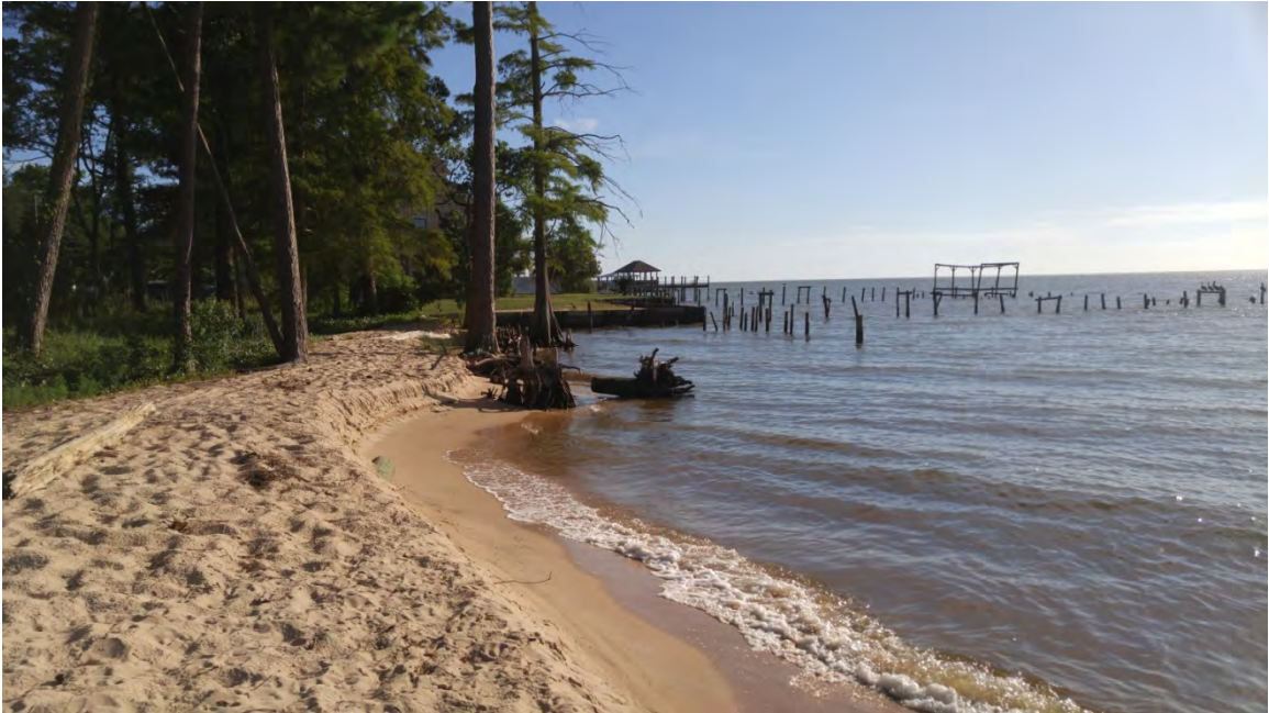
Figure 14: Photograph (facing south) showing summer erosion at the southern end of Magnolia Beach Park, near the American Legion (July 2016).
