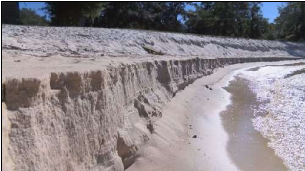
Pictured: An example of beach erosion in Magnolia Beach Park (Pier Street boat ramp area).
