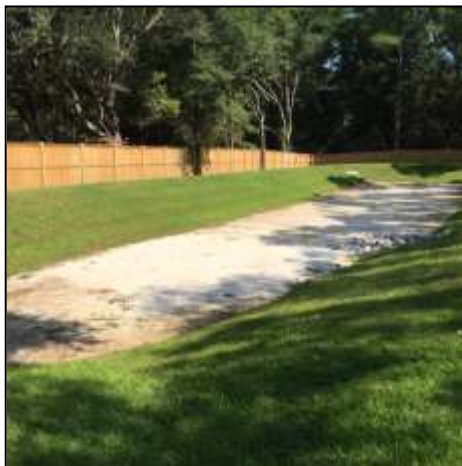
Pictured: Pointe Place subdivision stormwater facility (2015)
